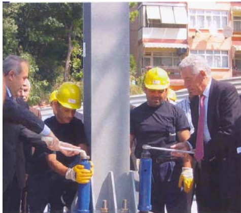
Erection of the first column by Erdal Ata (Province Governor) and Allan Collins (ECCS Chairman)
